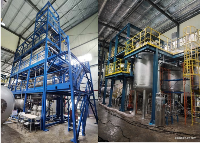
Distillation & LS mixing plant in ground hall
